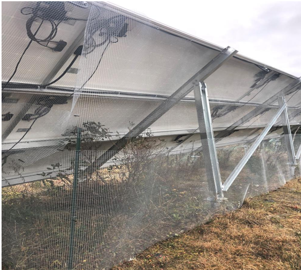
Photo 2: Example of unacceptable installation:
